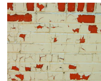
Painted porches are exposed to the elements and can peel and chip like this one (above).
